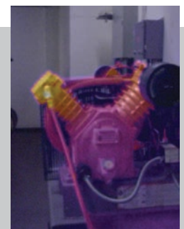
Air Compressor – AutoBlend™ Mode
