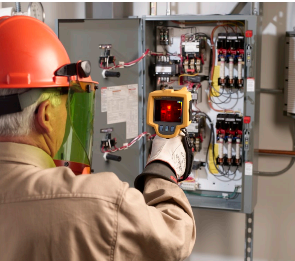
When scanning a live electrical panel, wear appropriate 70E personal protective equipment for arc flash and stand at least four feet away.
