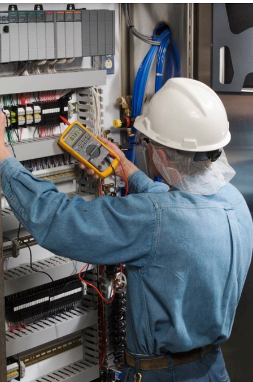
Keith Morin using his Fluke 787 Process Meter to spot-check ac noise on a 4–20 mA loop. The panel is an air-activated valve control center in the filter department of the plant, and it contains 120 V ac and a single 24 V dc power supply for 4–20 mA level sensors.
