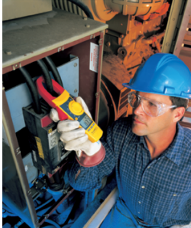
Figure 7: Measuring the loads on a power disconnect.
