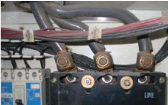
Figure 5: Three-phase power disconnect.
